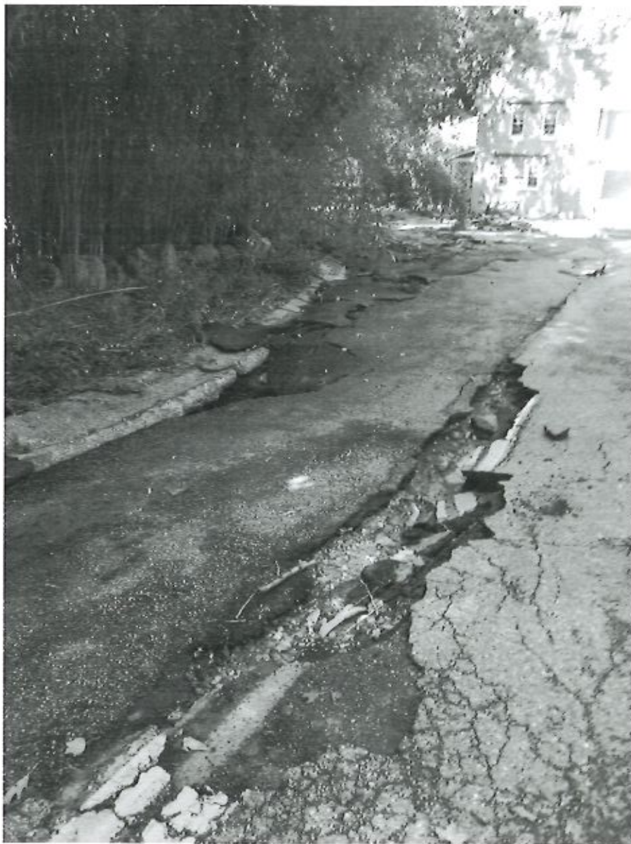
Some damage caused during Tropical Storm Ida due to overtopping of upper culvert.
