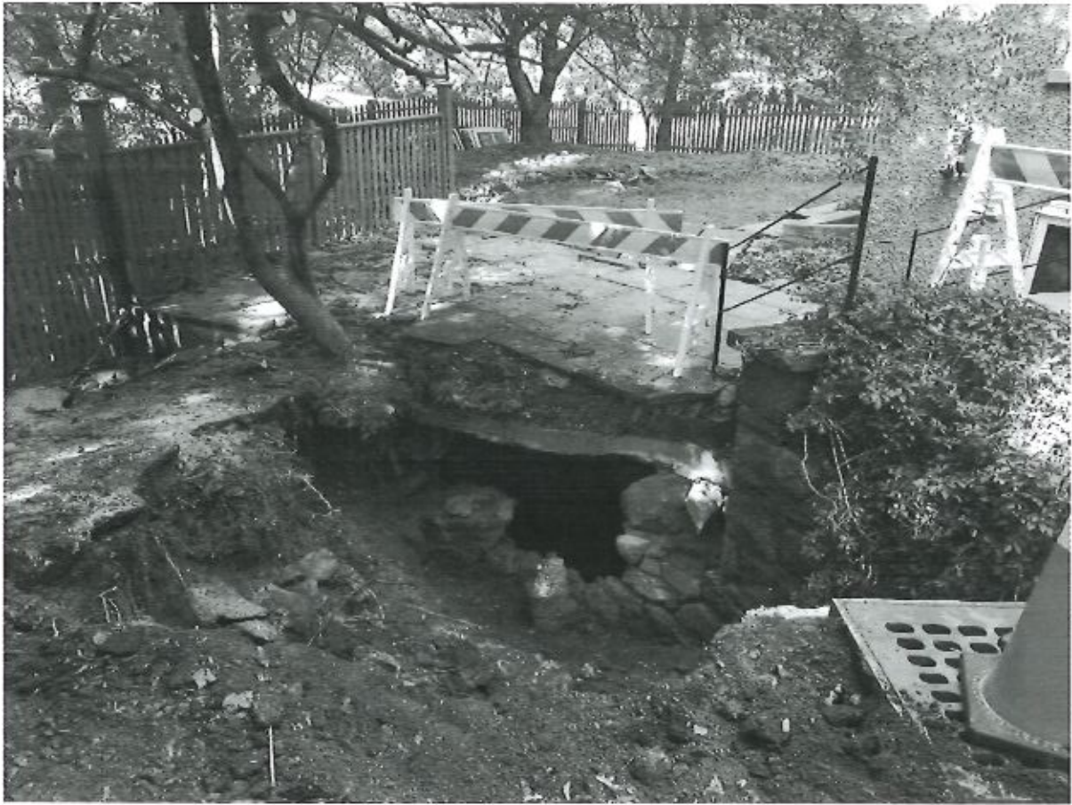
Lower culvert damage from Tropical Storm Ida
