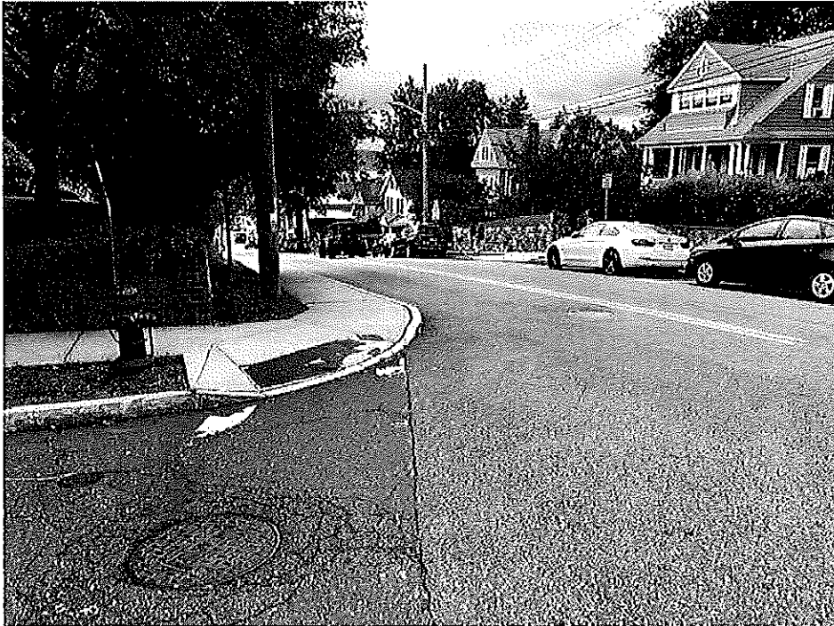
ADA ramp needs upgrading. Crosswalk needs re-stripping.
